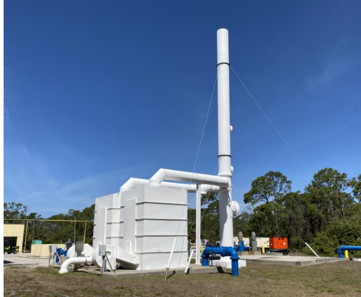
Photo 4-1: Existing RO Degasifier
