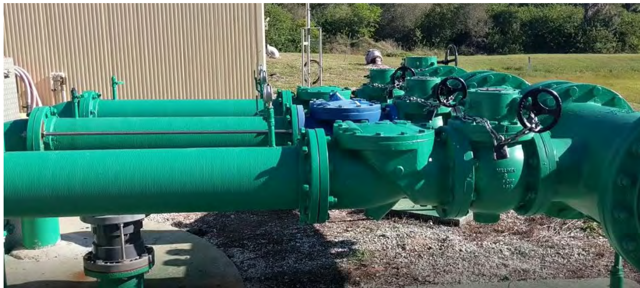
Figure 6: Existing Holiday Ventures Lift Station
