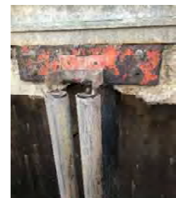
Figure 5: Pump Rail Plates on Missing Concrete
